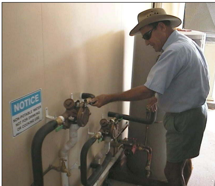
Plumbing Inspector David Massey checking the installation of backflow prevention devices at a new building construction
