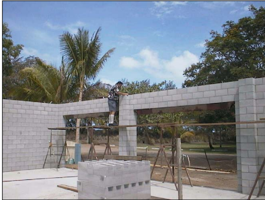
Building Inspector Trevor Maltby inspecting the bond beams at a new building construction
