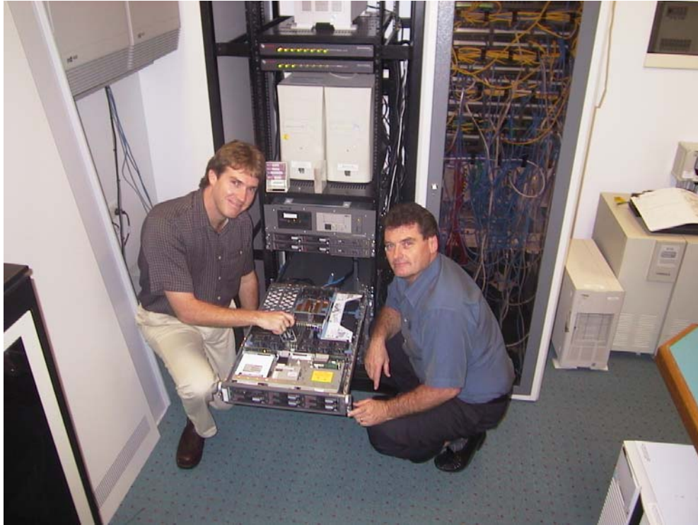
Information Technology Staff, Dirk Dabelstein and Battista Covolo installing new SQL Server
