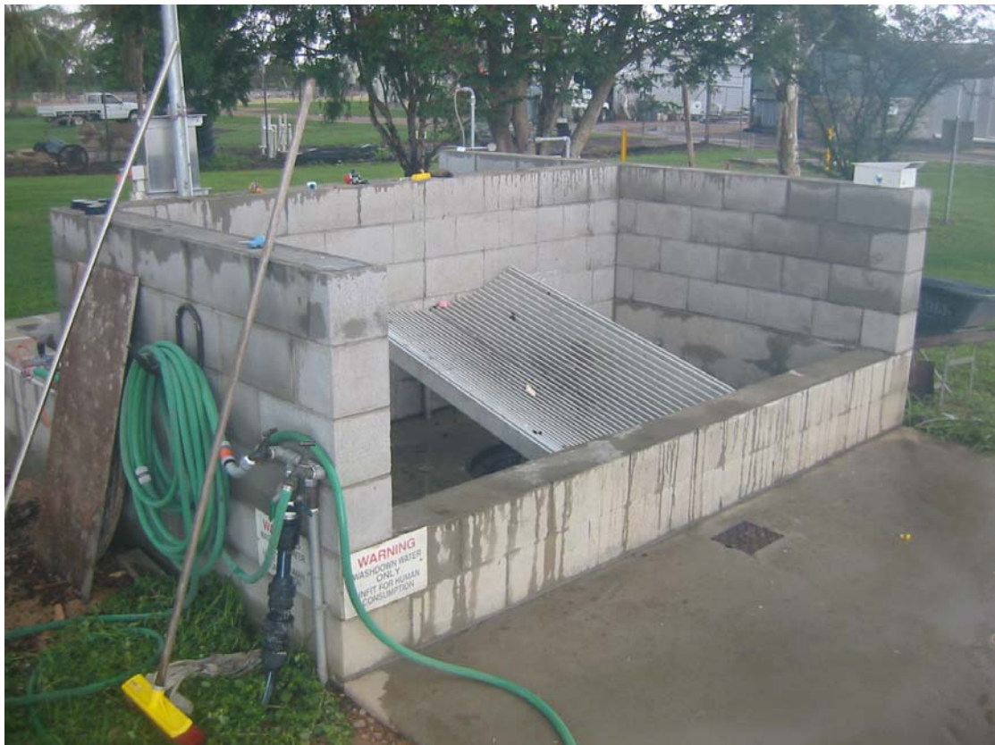
Improved Receiveal facility for septic tank sludge at the Ayr Sewage Treatment Plant.
