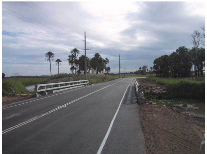
Completed works on new Bridge over Plantation Creek on the Rita Island Road.
