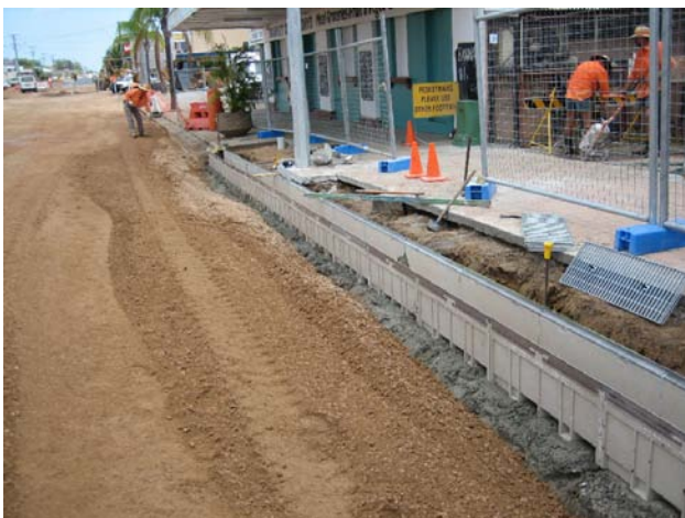
Burdekin Road Safety Audit – Edwards Street, Ayr - guttering
